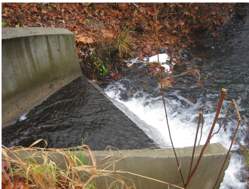
Woodhull Dam outfall prior to construction of fish passage. Photo credit: Peconic Estuary Partnership
