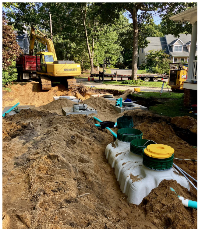
Installation of an Innovative and Advanced Water Treatment System (Fuji Clean CEN7) at a waterfront property in Suffolk County, NY. Photo credit: Bridgewater Environmental Services
