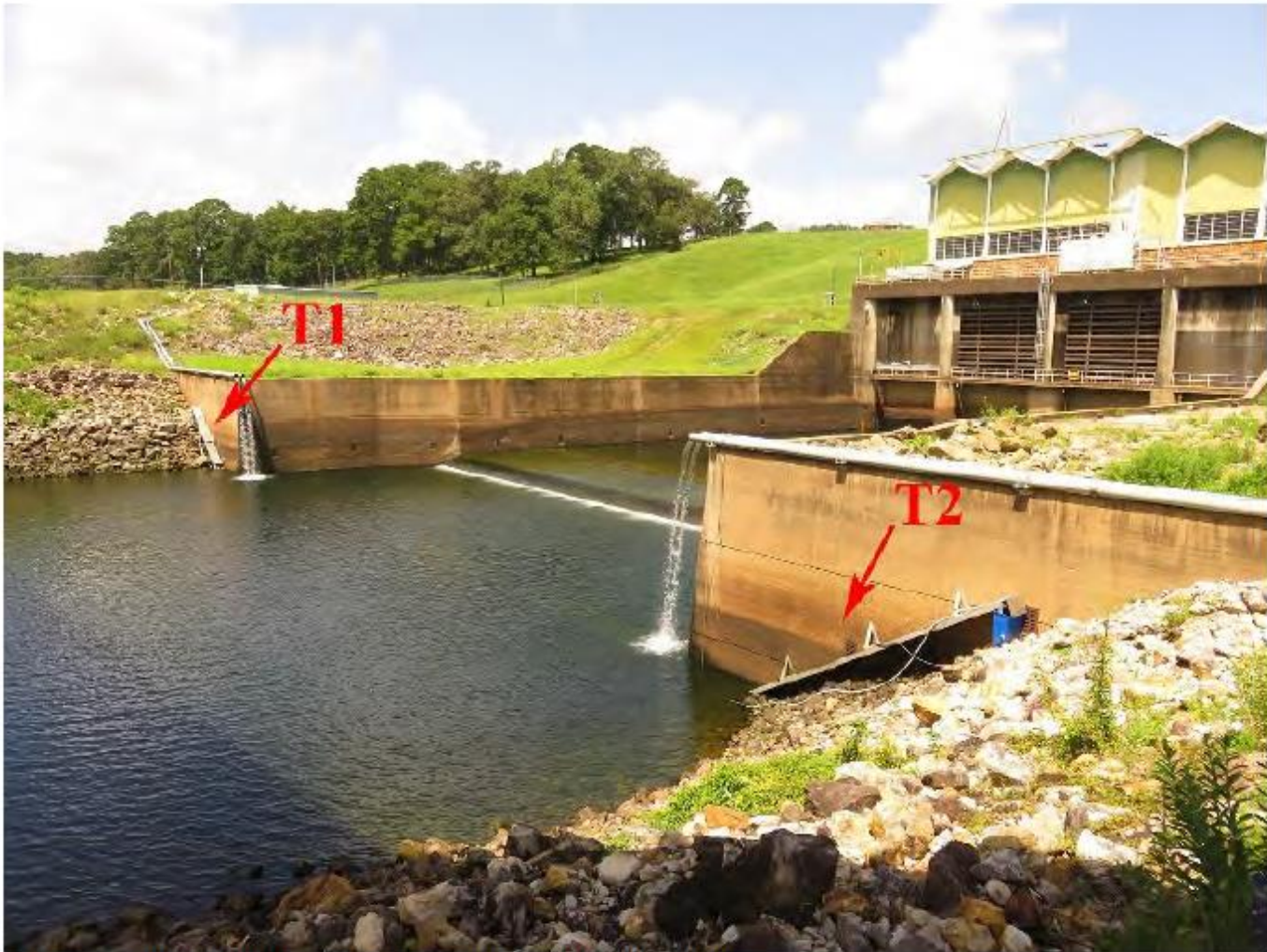
Figure 4. Toledo Bend Project Tailrace trap installations, non-generation
