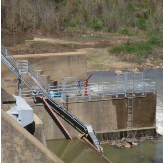
North Eelway 30M long, 43 degree ramp angle with two turn pools 250L holding tank → 350L spring 2018
