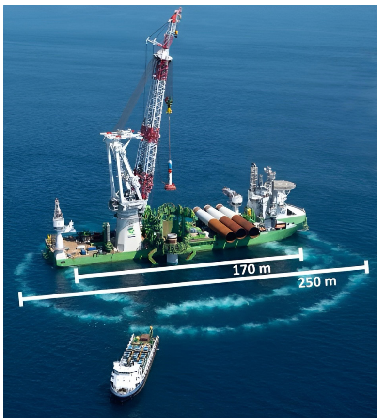
Bubble curtains are used during monopile foundation installation to, minimizing acoustic impacts to fish and protected species. Double bubble curtains are especially effective and can lower sound energy levels by up to 90%. Credit: DEME Group
