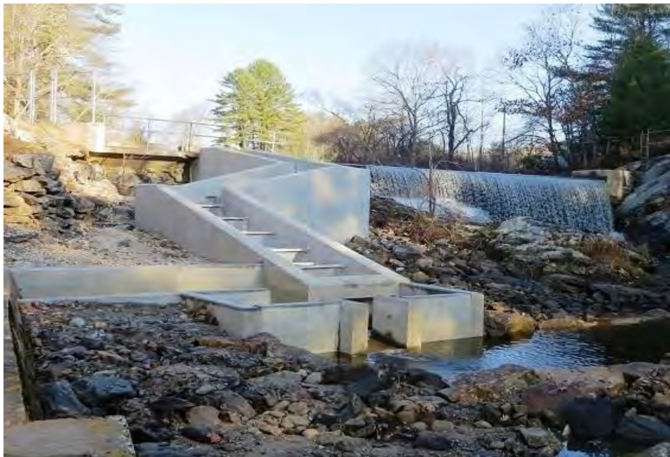
Figure 29. The Nequasset fishway and entrance to the trapping facility after repair in 2014.
