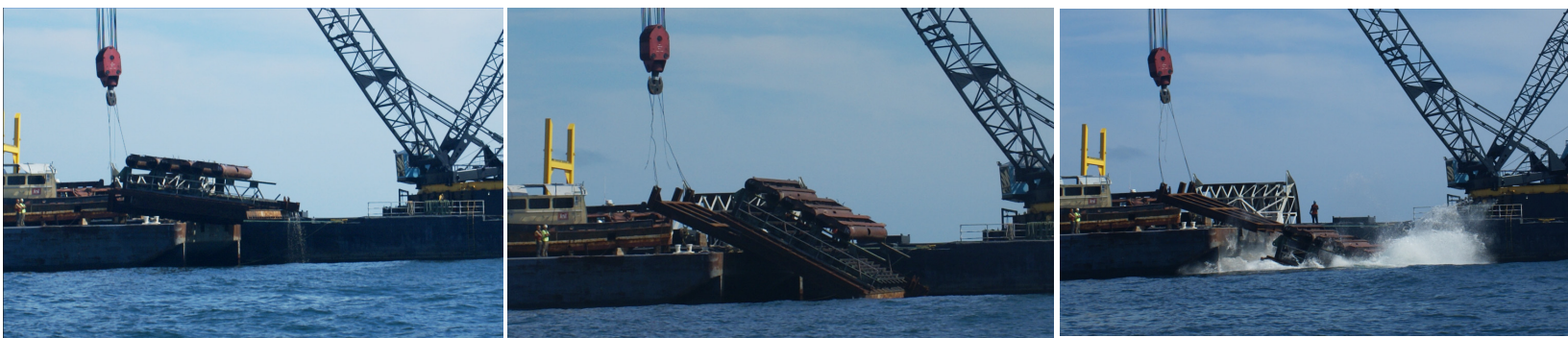
Figure 22. The deployment of the steel bridge/mitter gate/pontoon sculpture off the “slip and slide.” Photo credit: NYSDEC.
