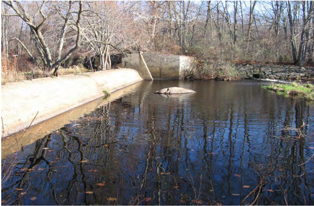
Figure 2: Photograph of the White Rock Dam, Dead End Channel at Low Flow Conditions
