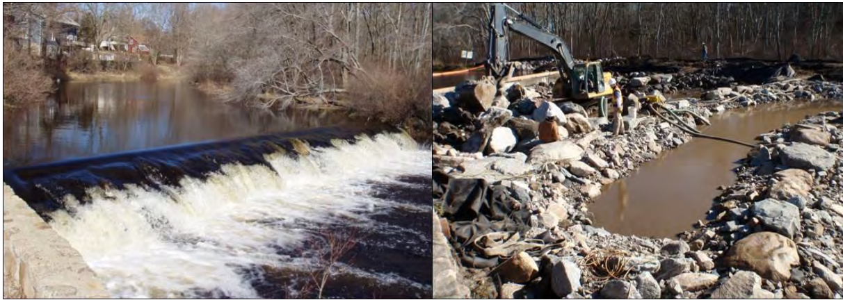
Figure C 20 – Kenyon Mill Dam, pre-removal (left – 2010) and NLF under construction (right – 2013). Credit: NOAA Fisheries.
