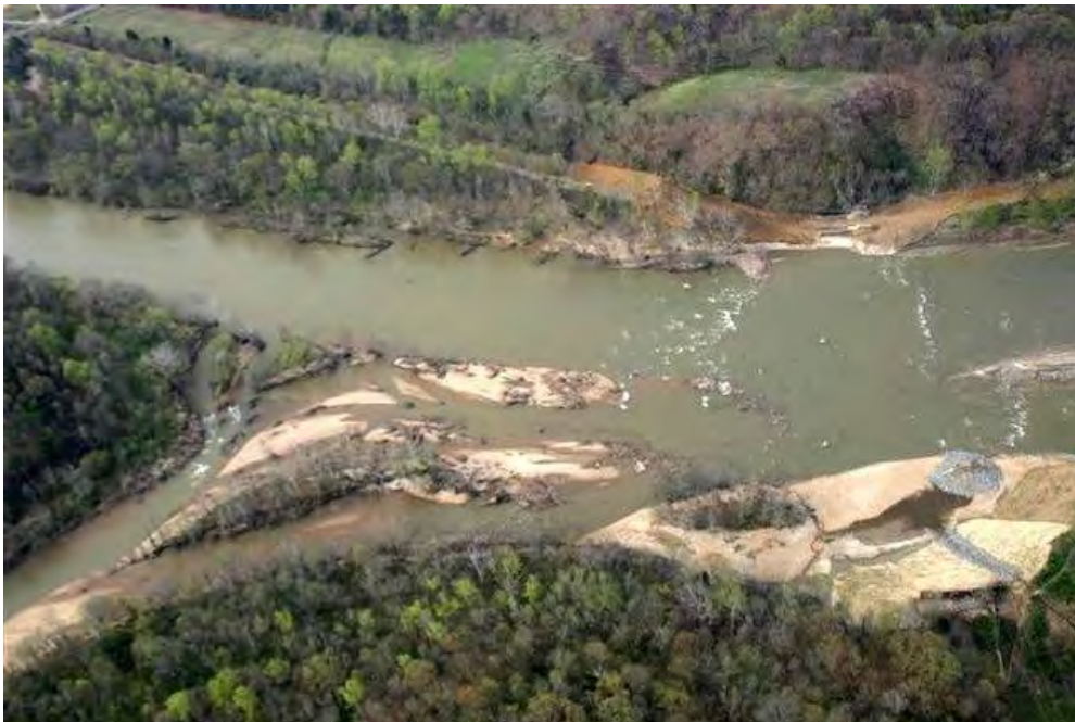
Figure C 42 – Aerial view of the restored portion of the Rappahannock River post-removal of the Embrey Dam. Credit: USACE.
