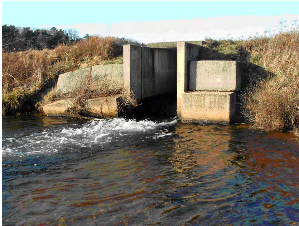
Figure C 9 – Middle Bog Dam, 2018. The Coonamessett structures were earthen dams with low-head concrete spillways and failing culverts that were effective as herring passage barriers. Credit: Town of Falmouth, MA.
