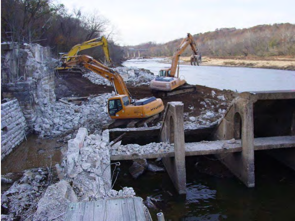
Figure C 41 – Mechanical removal of the remaining structural pieces of the Embrey Dam. Credit: Alan Weaver/ VADWR.
