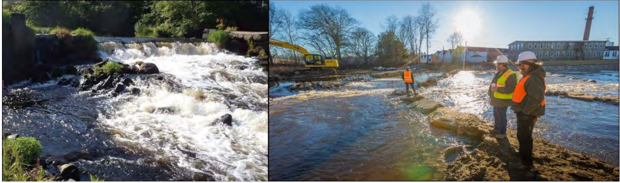
Figure C 22 – Bradford Dyeing Dam pre-removal (left) and installation of NLFs (right) in 2017. Credit: NOAA Fisheries (left) and Ayla Fox/TNC (right).
