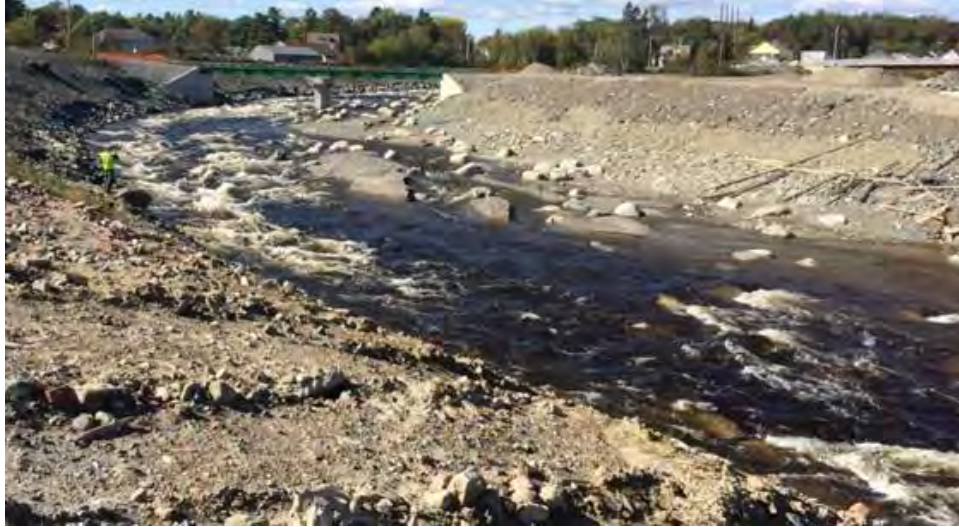
Figure 7 – Howland Dam bypass nature-like fishway on the Piscataquis River in Howland, ME. Credit: NOAA Fisheries.
