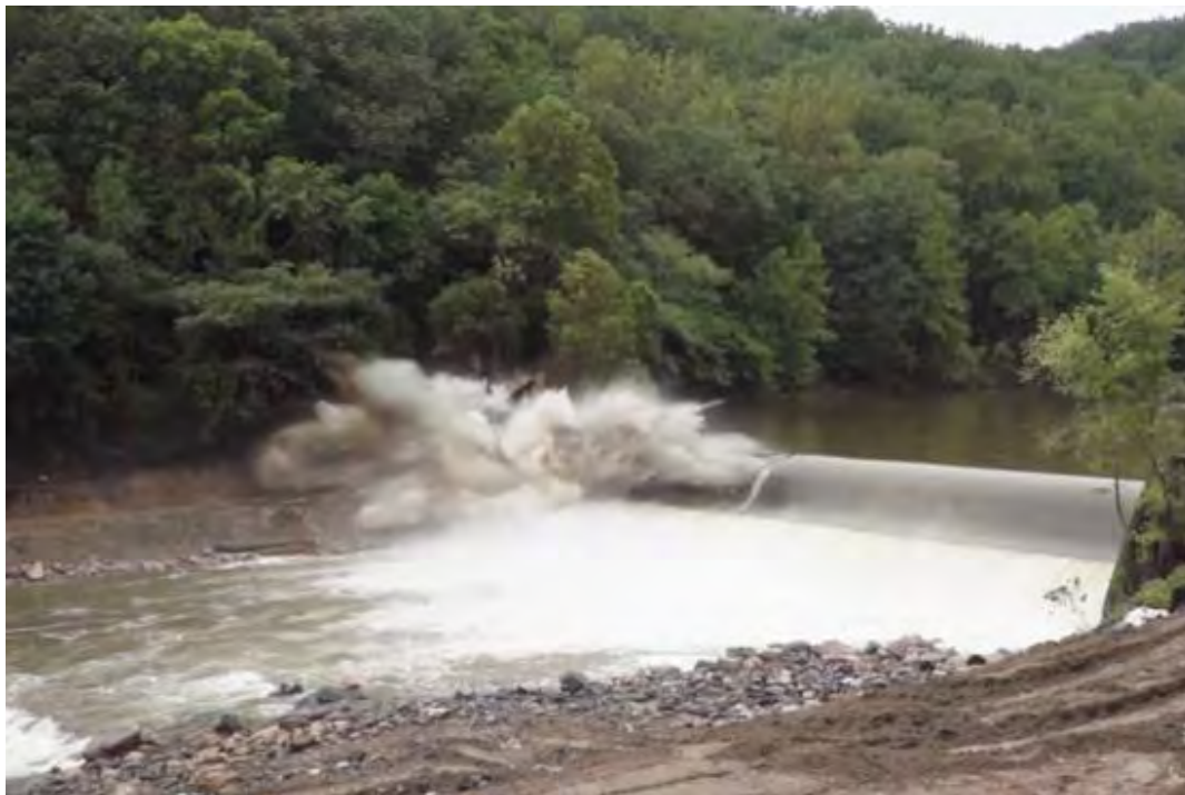
Figure C 34 - Initial Breaching of the Bloede Dam via explosives Credit: Elevate Media, Inc. and MDNR.
