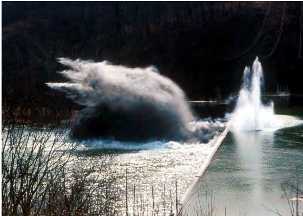
Figure C 39 – The second explosion set off during the demolition day event to breach the Embrey Dam. Credit: VADWR.
