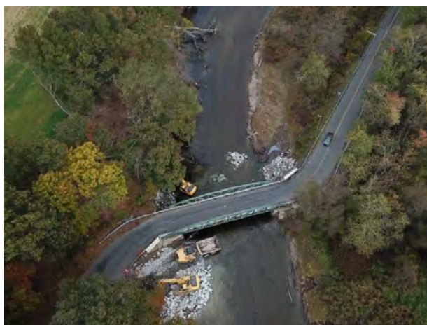
Figure C 32 – Warrington Bridge scour protection, view from above. Credit: Dave Zuckerman/ Columbia Volunteer Drone Team.
