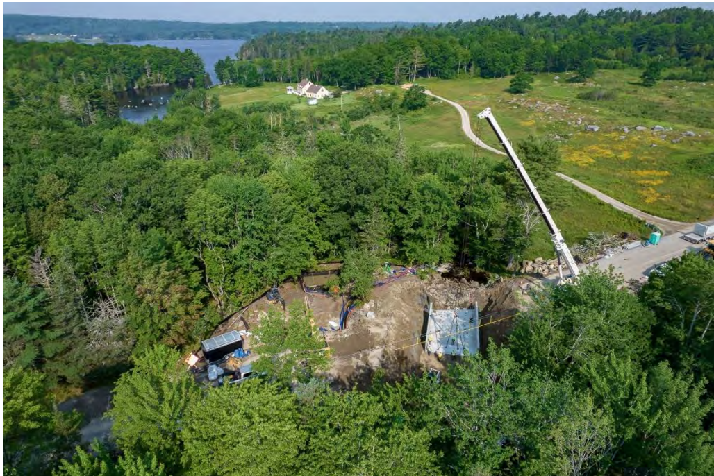
Figure C 5 – Aerial view (perpendicular to road) of the construction site for the installation of a large box culvert on Snow's Brook. Credit: Ken Woisard Photography/ MCHT.
