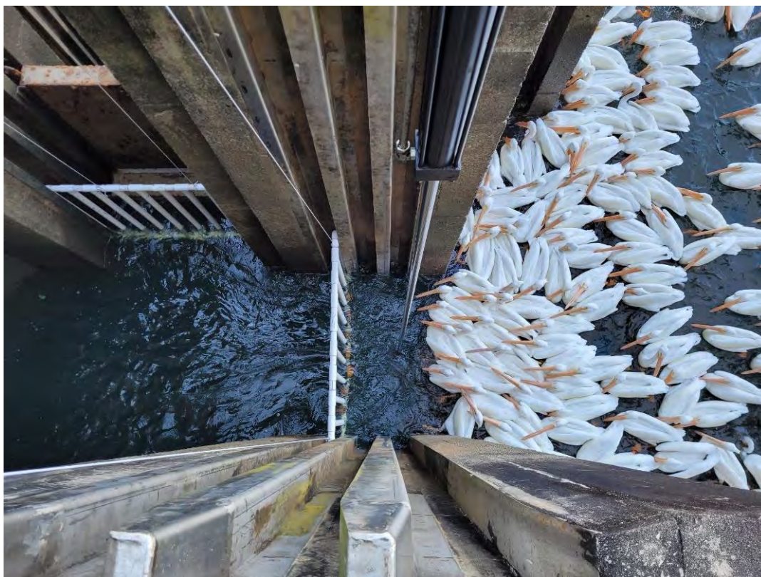
Figure 10 – Temporary exclusion installed for white pelicans on the St. Stephen fish lock and dam in the Santee River, SC. Credit: USACE.
