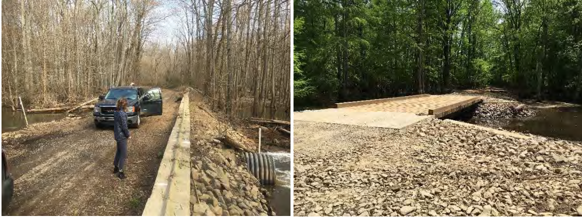
Figure C 46- Phase 2 crossing with culvert (before, left) and bridge (after, right). Credit: Aaron McCall/ TNC.
