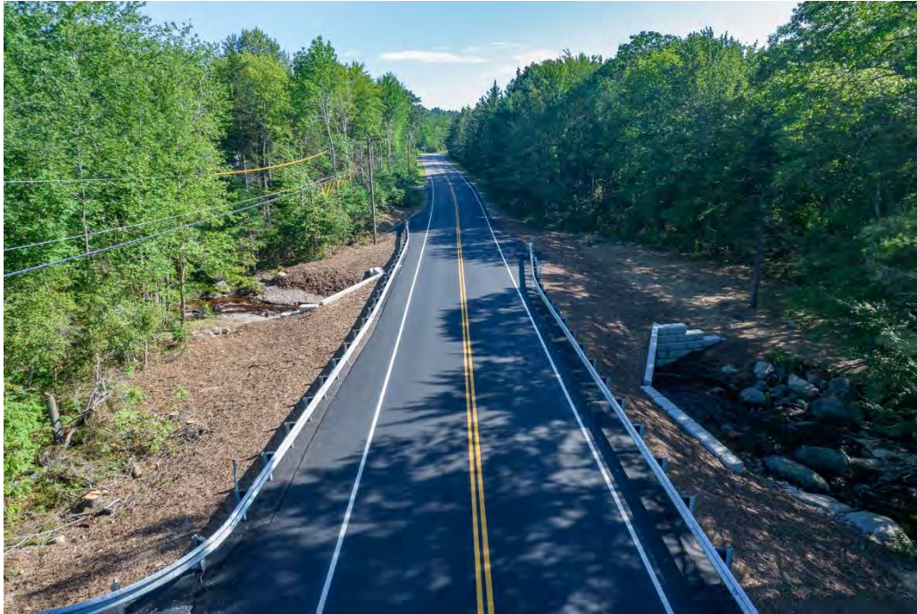
Figure C 6 – Aerial view of fully installed box culvert on Snow’s Brook. Credit: Ken Woisard Photography/ MCHT.
