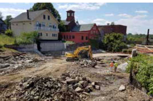
Top left: Attached fish ladder demolition; bottom left: Dam removed; river restoration commencing Photo credit: NH FGD
