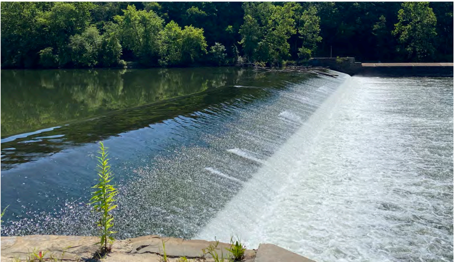
Black Rock Dam on the Schuylkill River, in southeastern Pennsylvania. Image credit: TNC.
