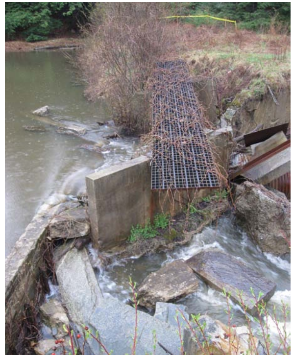
Perched culvert on Shoreys Brook
