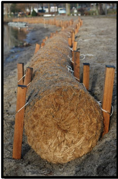
Figure 20: Example of a living shoreline stabilizer called biodegradable organic natural fiber logs (biologs) (Photo credit: Maryland Department of Natural Resources)
