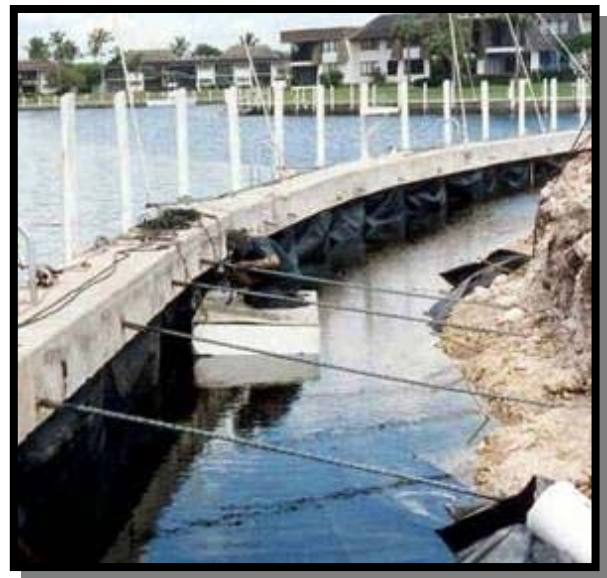
Figure 6: Seawall developed seaward of an eroded shoreline (Photo credit: Florida FWC)
