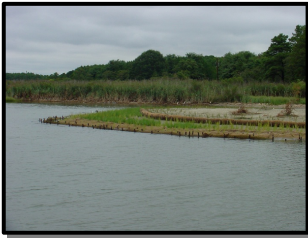
Figure 2: Living shoreline stabilized using sand fill and dredge material, coir fiber logs, wetland plants, submerged aquatic vegetation, an oyster reef breakwater, and fish habitat structures at Horsehead Wetlands, Chesapeake Bay, Maryland. (Photo credit: NOAA)
